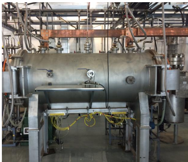
Fig. 6 Photo of the radiative heating system.
