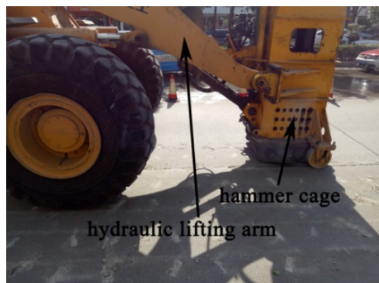
Figure 1. Micro-crack homogenization crushing of pavement structure [2].
